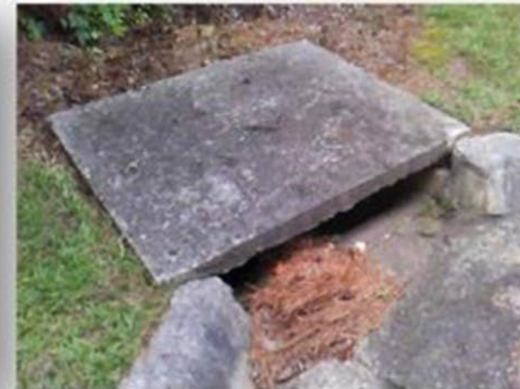
Inaccessible Catch Basin Lid
